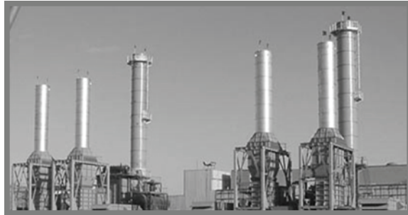
Gas-Fired Turbine Peaker Plant
