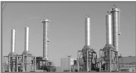
Gas-Fired Turbine Peaker Plant
