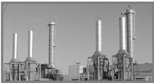
Gas-Fired Turbine Peaker Plant
