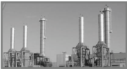
Gas-Fired Turbine Peaker Plant
